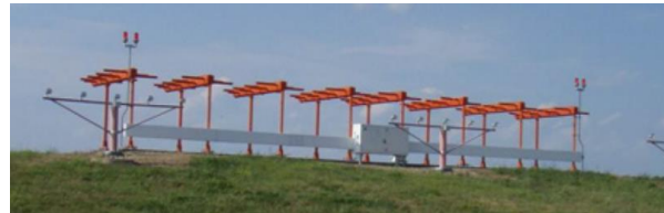
Typical Localizer Antenna Array (FAA)
