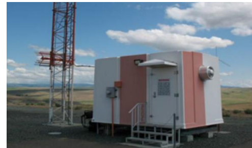
Typical Glide Slope Antenna (FAA)
